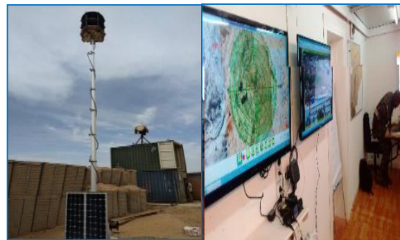
Fig. 14. Ground radars and public address warning (PAW) system in Kidal camp and Mopti camp, MINUSMA
